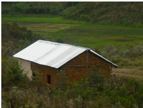
Fig. 6. The primary school in the village of Ranomainty, Didy Commune, in Nov 2012, repaired following damage by Cyclone Giovanna. (Photo: Lucien Randrianarimanana)
